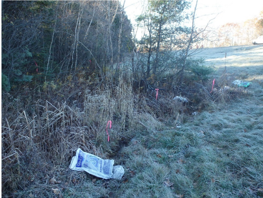
Photo 3. Wetland C: PEM/PSS, closed, depressional wetland along roadside toe of fill; outlet of culvert from Wetland D. Stantec, November 9, 2017.
