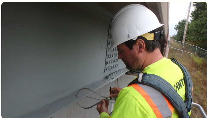
Photo 22: Bennett Road Bridge Section Loss Measurements
