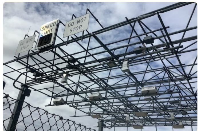
Photo 12: Toll Equipment (Spaceframe Infrastructure)
