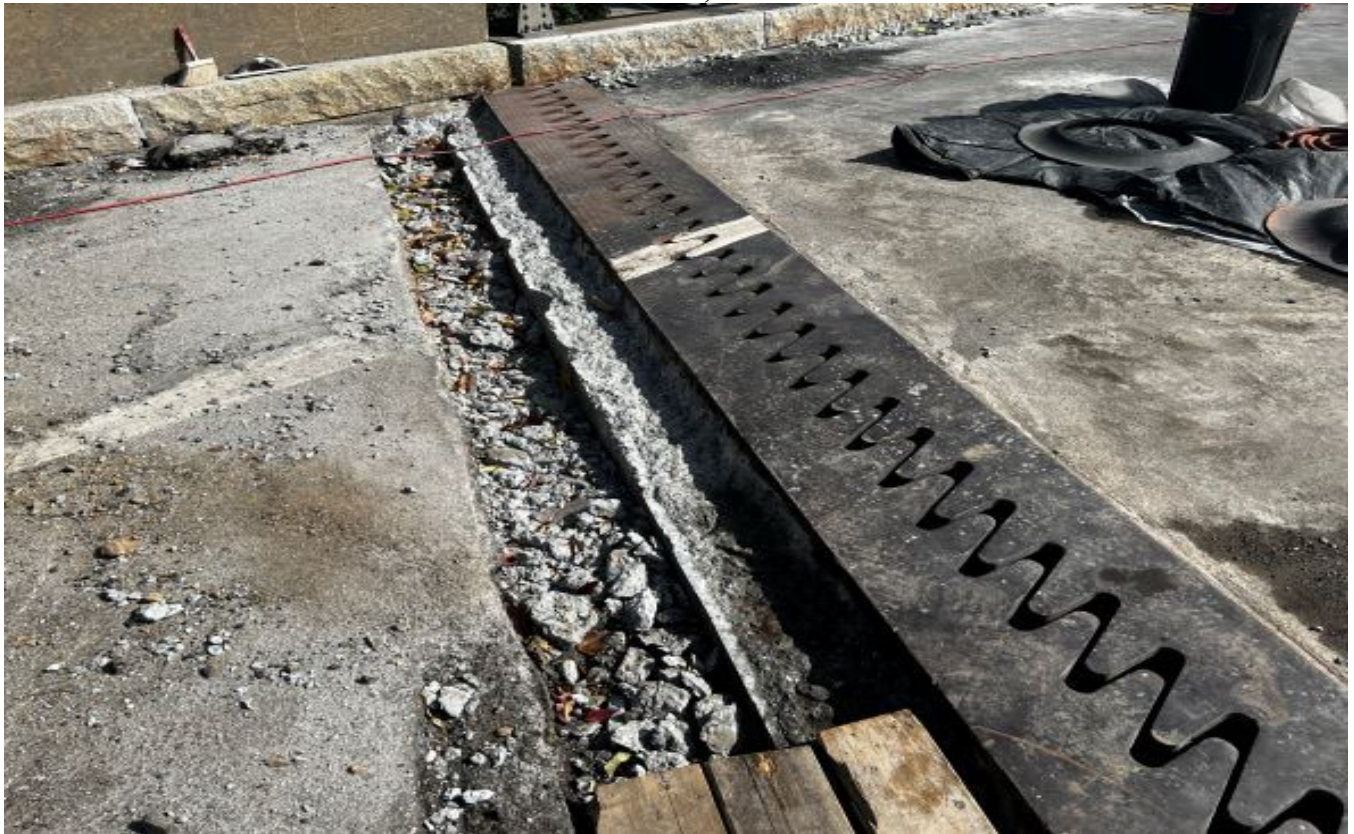
Ramp H looking at the west bridge approach. Repairs to the adjacent concrete at the finger joint.
