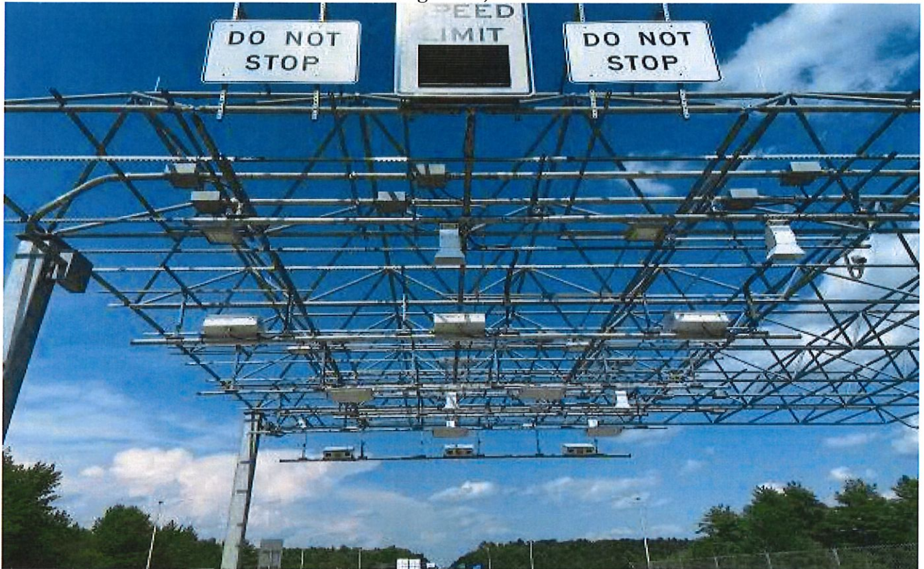
North bound ORT space frame showing the updated sensors and transponder readers.
