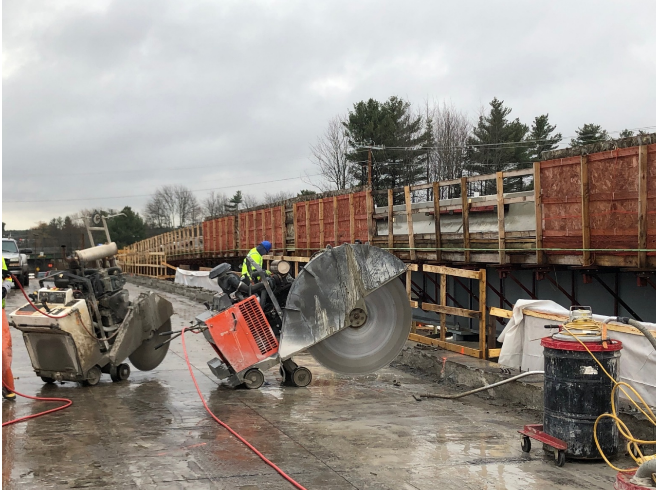
Saw cutting deck for removal. Notice new bridge is higher than the old bridge.
