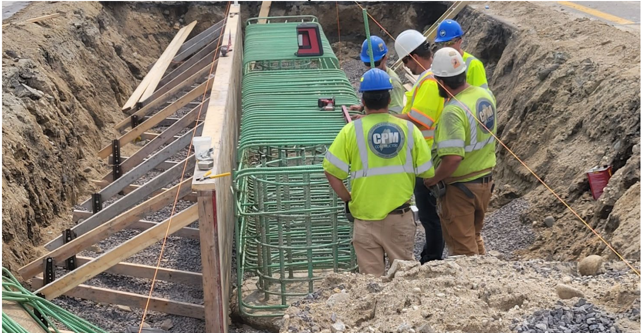
Project leadership reviewing the reinforcing steel for the Overhead Sign Structure Foundation
