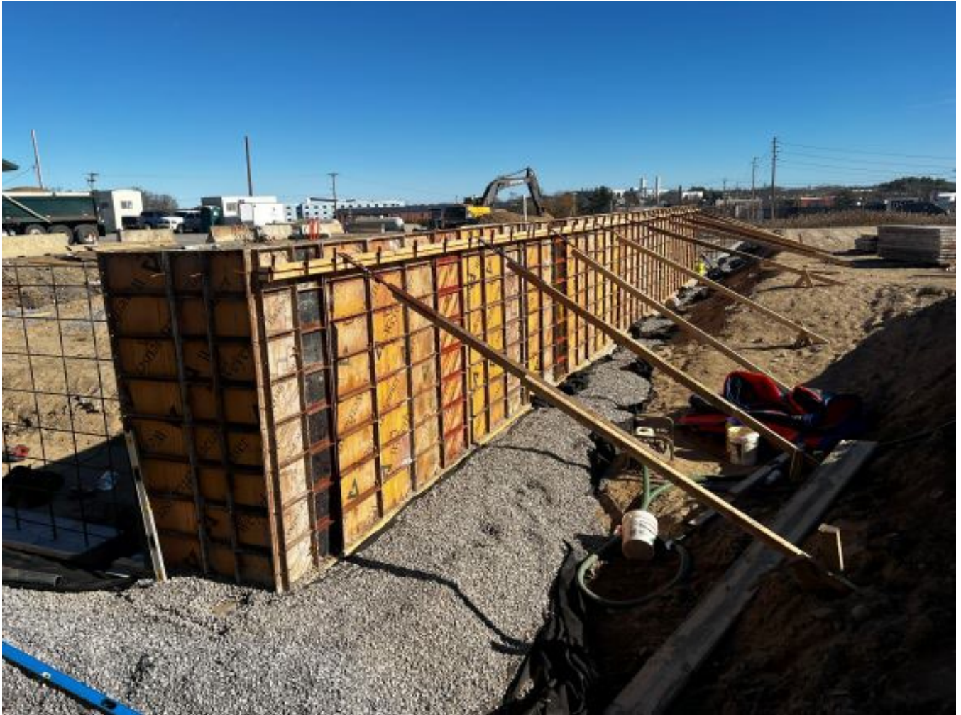
Concrete formwork for the backside of the foundation to the new 8 bay vehicle storage building.
