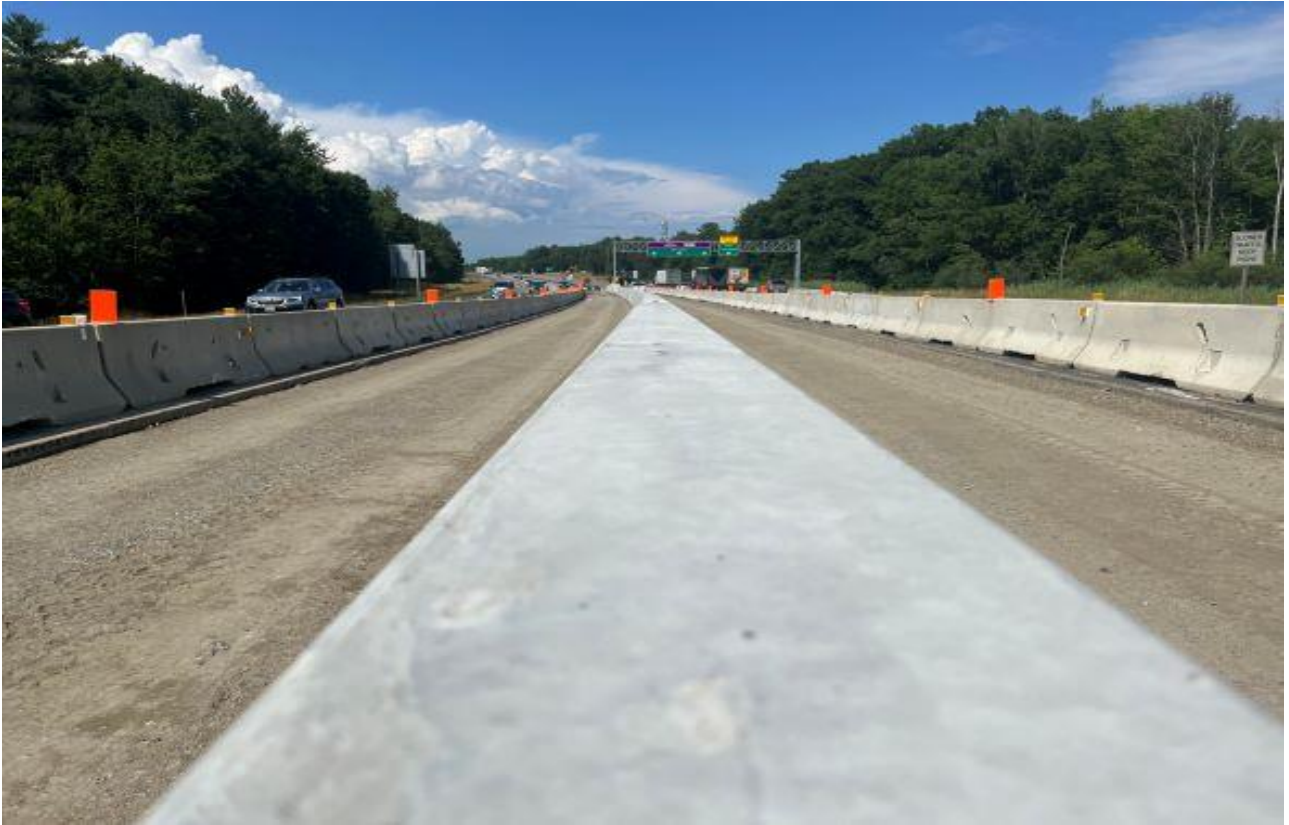
Looking north in the median, Sargent crews are prepping gravel for pavement adjacent to the concrete barrier.
