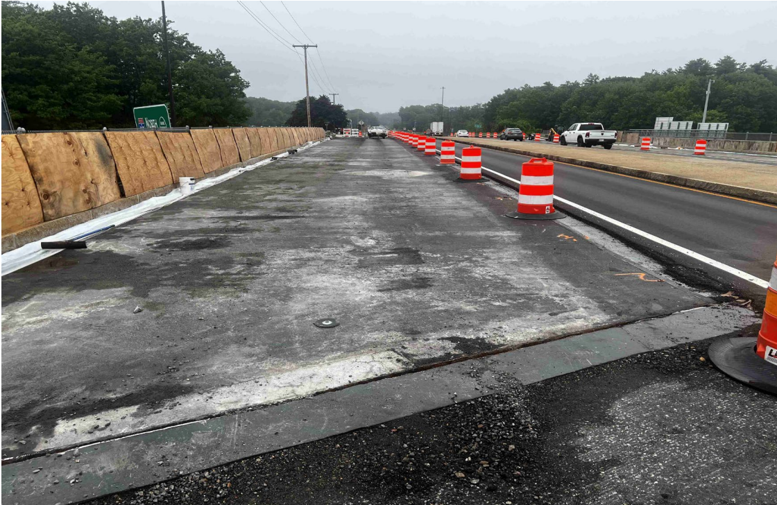
Looking west along the east bound lane of 236. Minor concrete repairs along the gutter line only.
