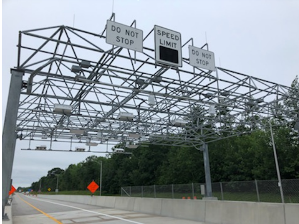
South bound West Gardiner Barrier Toll Plaza with the new equipment installed.
