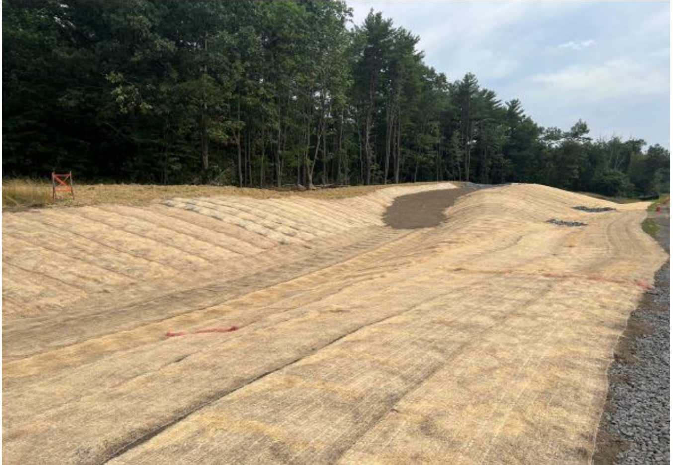
Looking south at the northbound stormwater treatment system that was recently constructed.
