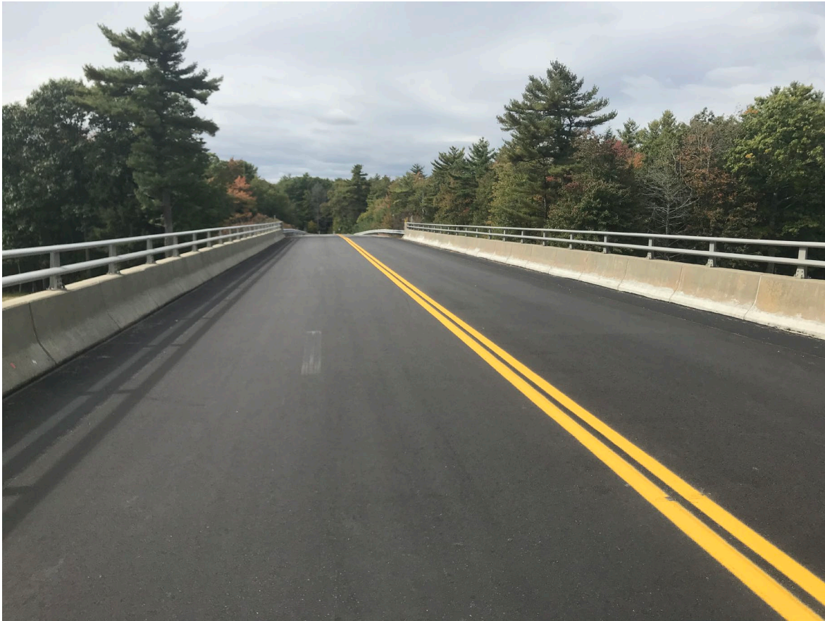
Mountain Road Bridge with a new wearing surface, striping, and concrete repairs.
