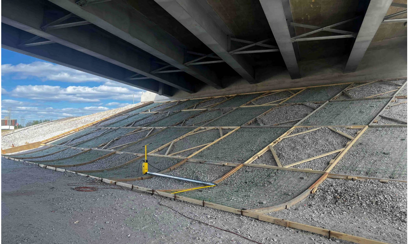
Slope protection formwork under the north bound side of the new Exit 45 bridge.
