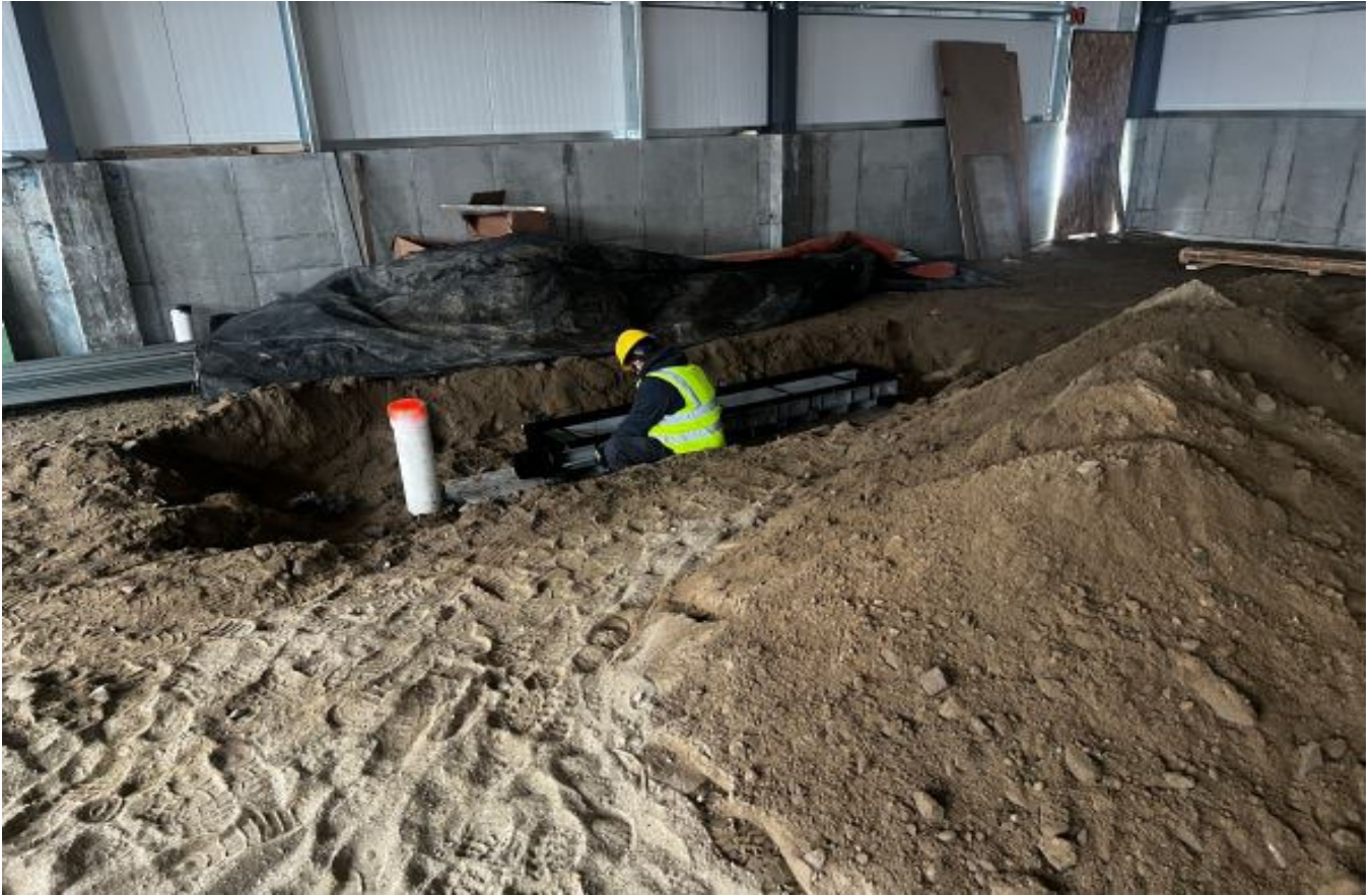
Looking west inside the new 8 bay garage. One of the floor drains being installed.
