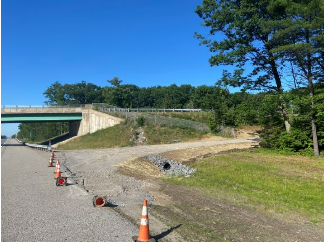
Burnt Mill Road NB EVR ramp. A-Gravel has been installed and is awaiting pavement.
