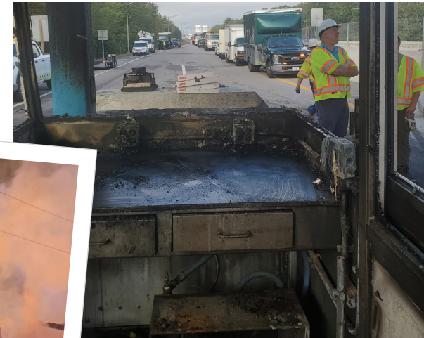
Destruction from inside booth
