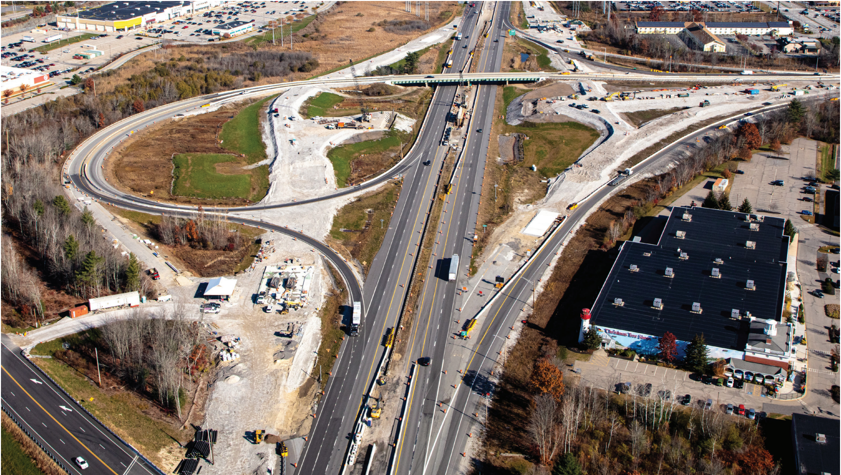
Exit 45 in November as CPM Constructors worked on interchange ramps and toll plazas
