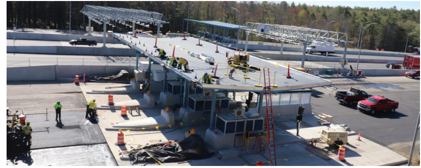
Reed and Reed and their subcontractors work on the southbound toll booth canopy in May
