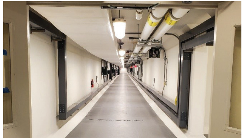
The new tunnel under the ORT is dry, well-lit and roomy for all of the new electronic equipment and for our toll collectors.
