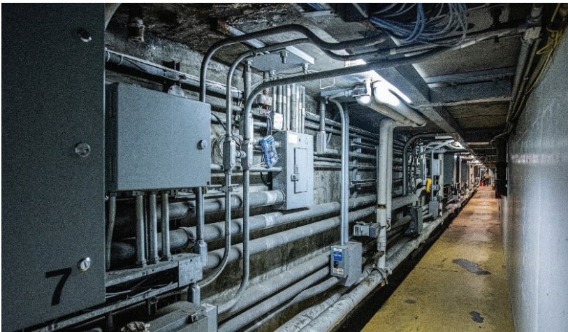
The tunnels under the toll booths not only serve as way for employees to get to their booths but also house all of the electronics for the booths and the toll collection system, here is what the tunnel under the old plaza looked like.
