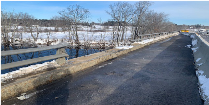
SACO RIVER OVERPASS (SB) RAILING COLLISION DAMAGE
