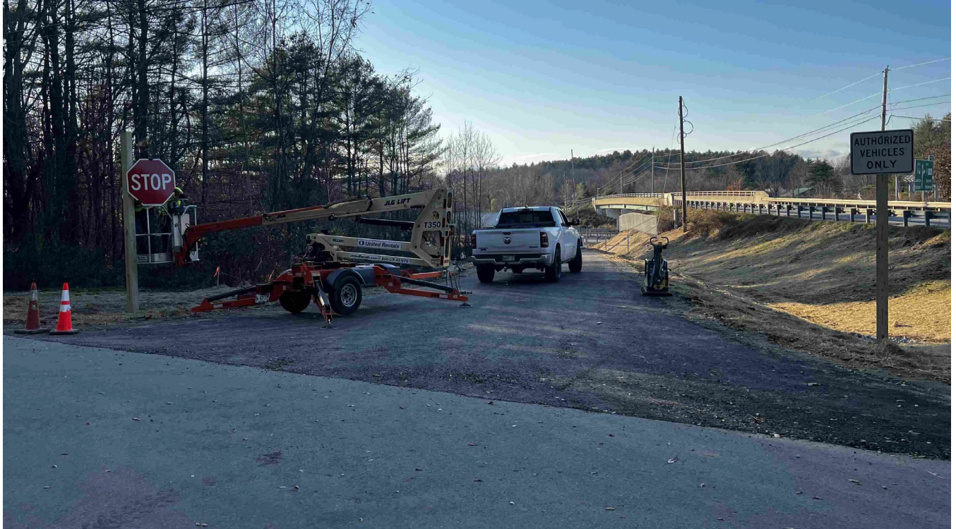
Looking at the north bound EVR from Terri Lane, crews are installing a stop sign.
