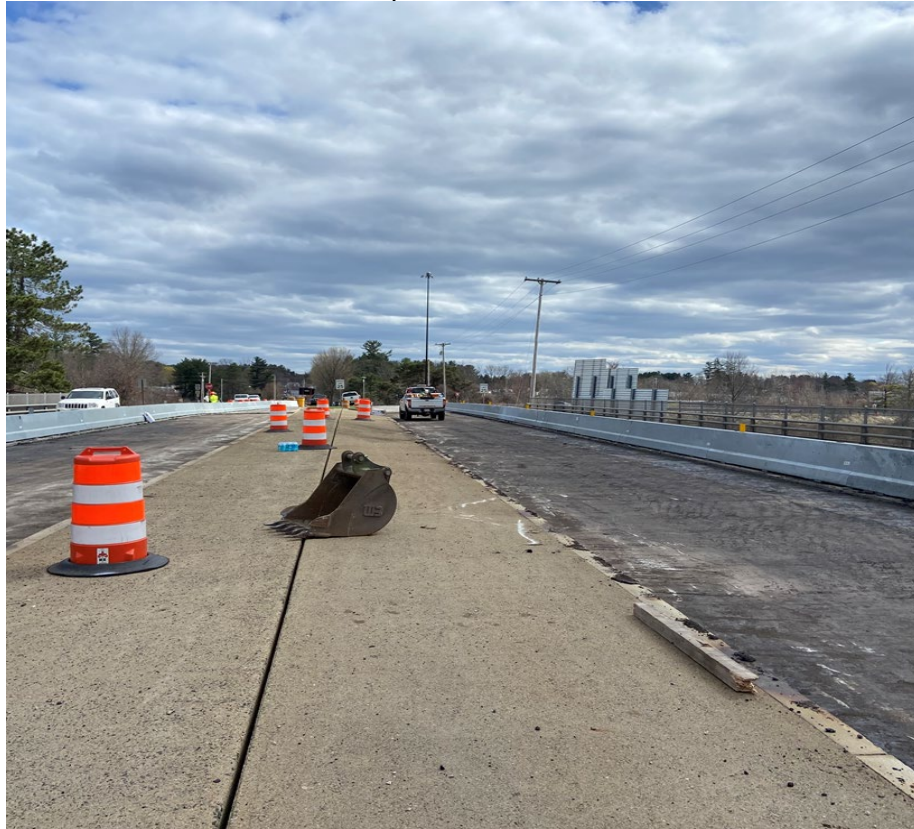
Route 236 bridge looking at the center median: bridge deck stripped of wearing surface.
