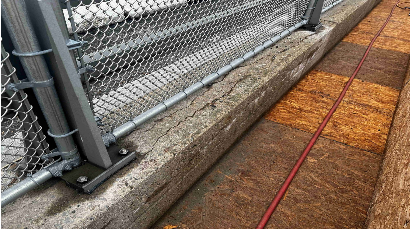
The north curb of Wilson Road showing areas of unsound concrete.
