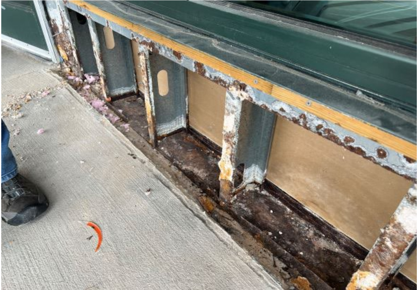
Rusted out framing at the northbound Kennebunk Service Plaza.
