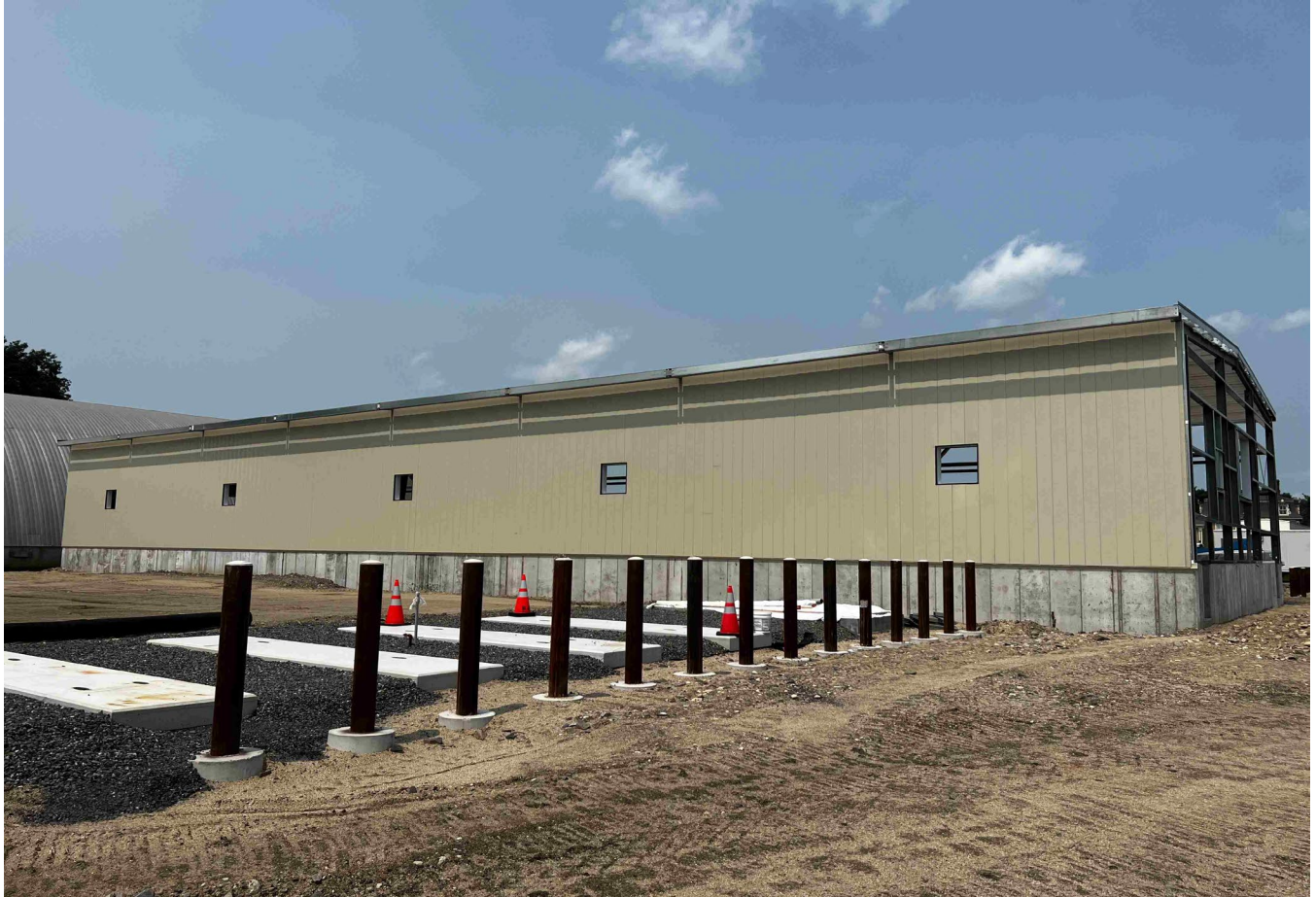
The backside of the new 8-bay. Bollards for the propane tanks in the front.
