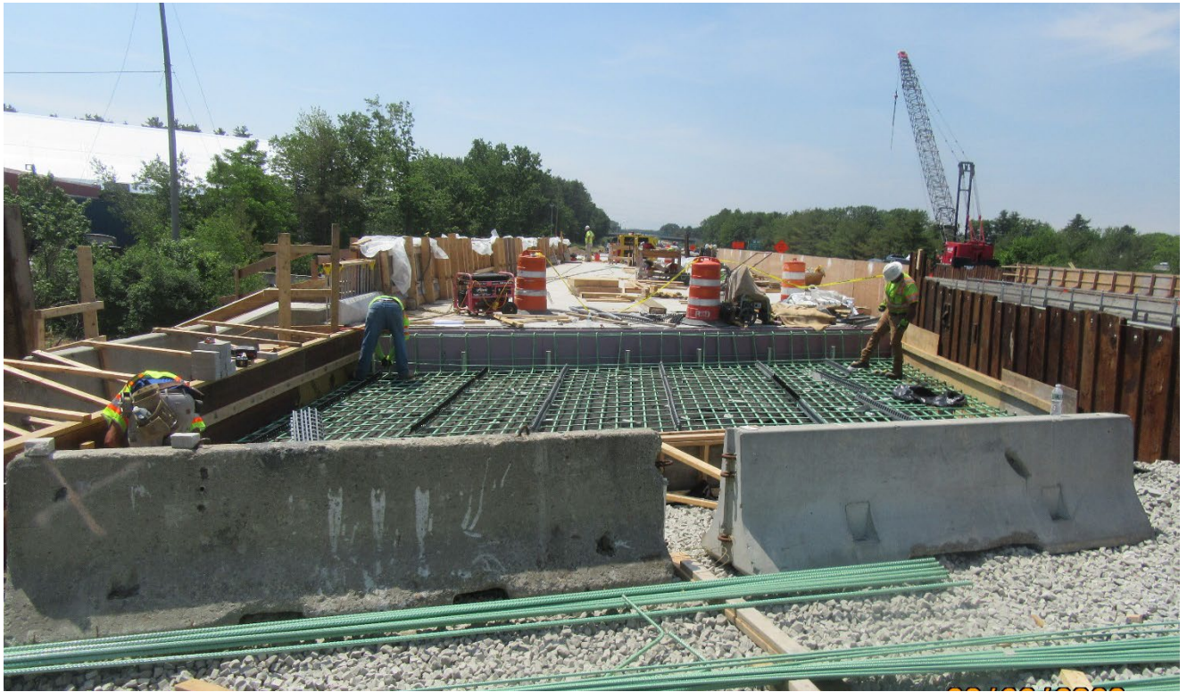
Crew tying reinforcing steel for the north approach slab at the northbound bridge
